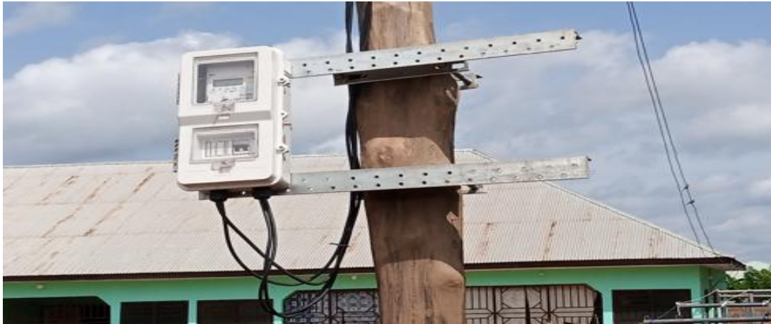
Fig. 1- shows a picture of a smart meter fixed on a pole.
