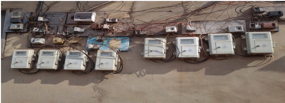
Figure 5b shows multiple prepaid power meters on a wall.
