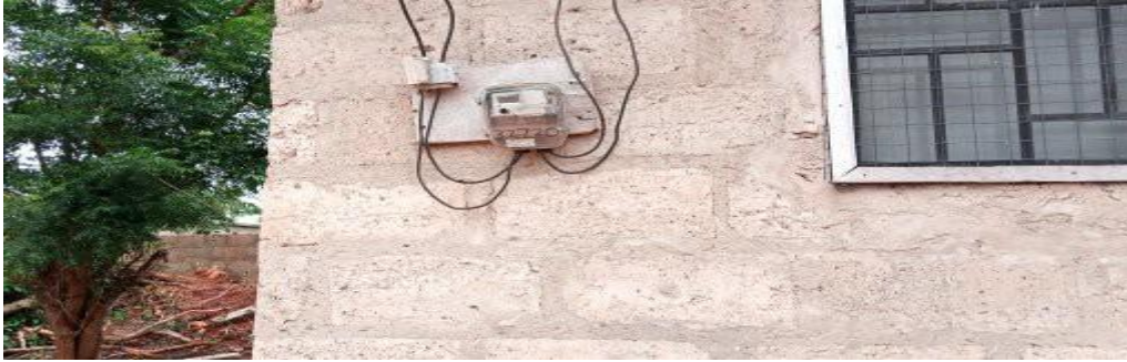
Figure 5a. A postpaid power meter.
