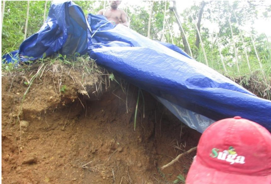
Figure 2. Landslides at the location behind Mr. Dani's house
